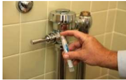
Toilet flush handle
