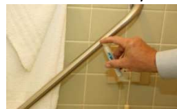
Toilet hand holds / rails
