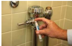
Toilet flush handle
